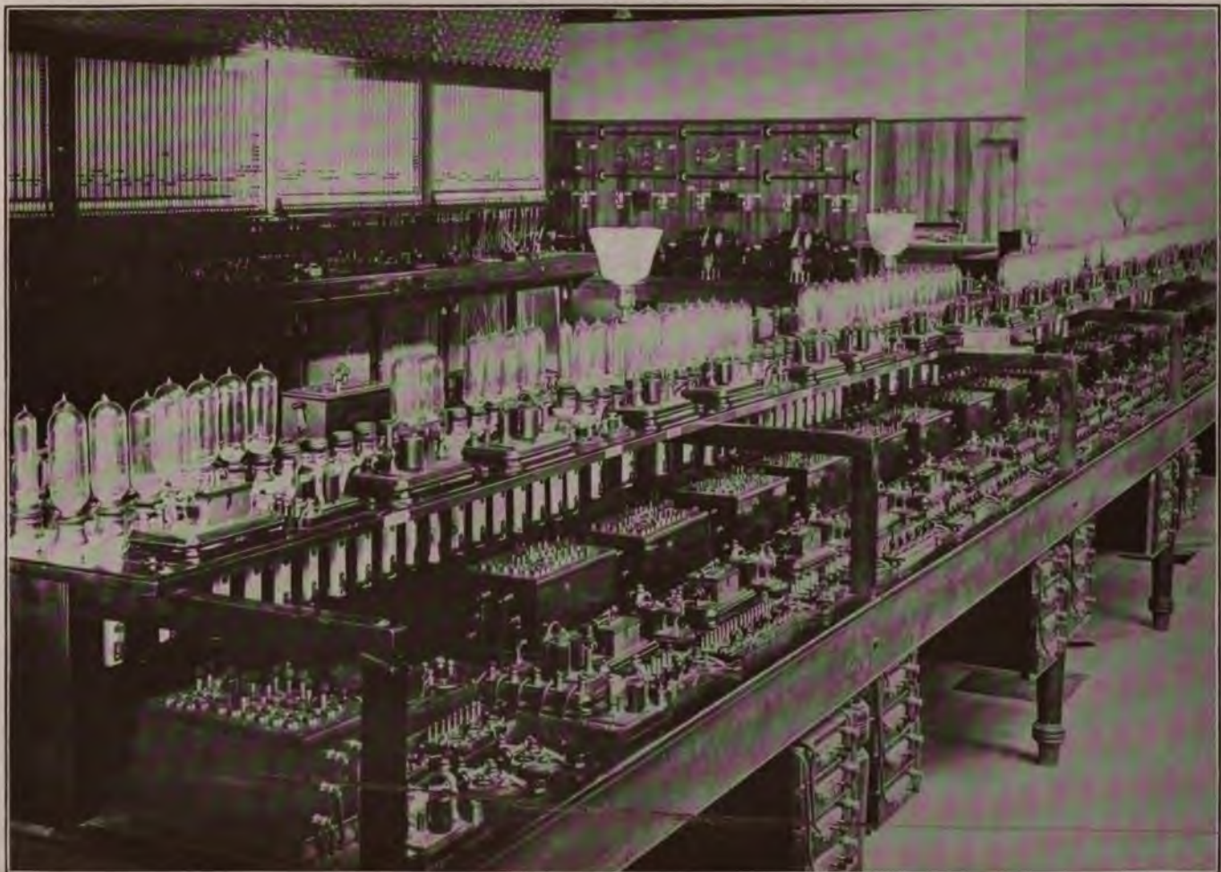
AUTOMATIC REPEATER EQUIPMENT IN TELEGRAPH OPERATING ROOM.
